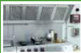
Commercial Kitchen Suppression Systems
